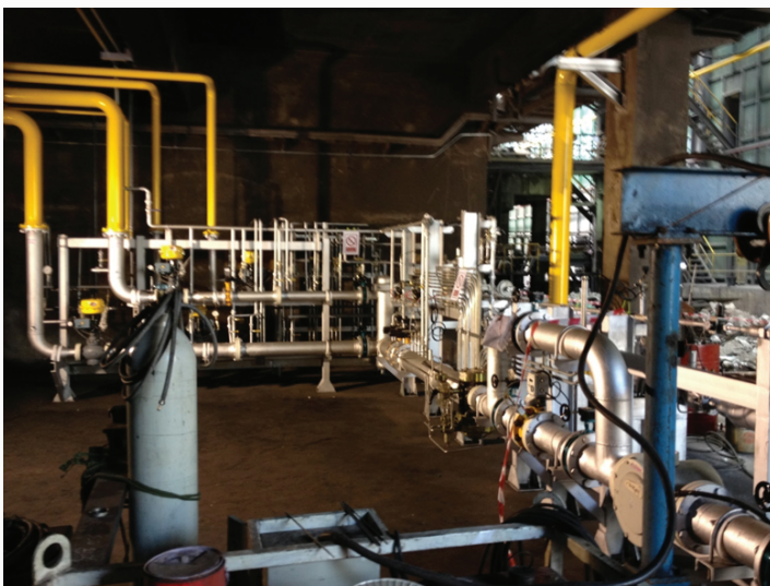
Natural gas piping
