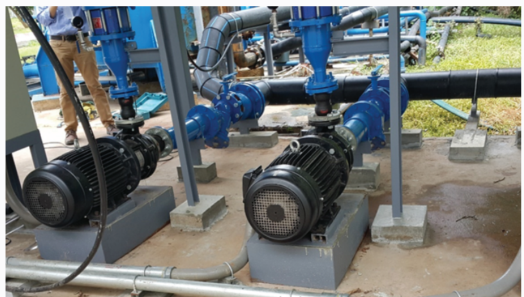
Automatic booster pumps and PE piping
